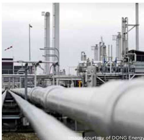
The Danish Stenlille Gas Treatment Plant where Ramboll has designed all above-ground facilities and thereby securing gas supply for the Copenhagen metropolitan region.
