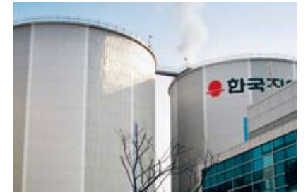
Ramboll has carried out several studies for the Korean District Heating Engineering Company, including an analysis of a new district heating transmission line between two power stations.
